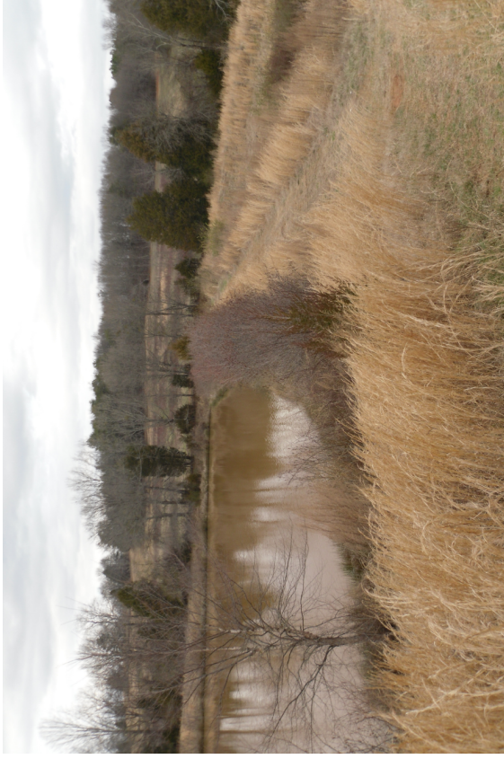
1: Thick vegetation on the upstream and downstream slopes of the dam
