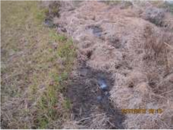
seepage at toe of channel
