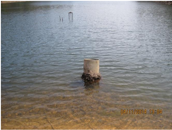
Trash rack w/ debris
