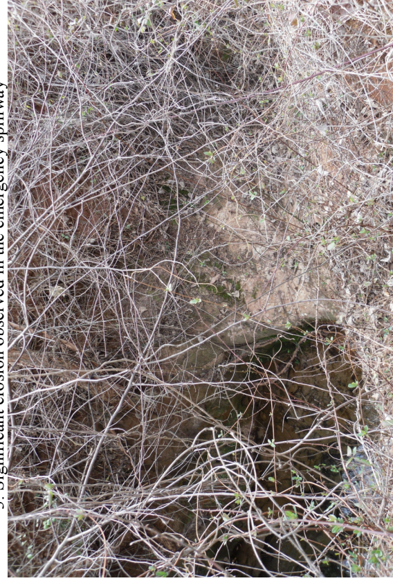
4: Large gully/ area of erosion between outlet pipe and emergency spillway
