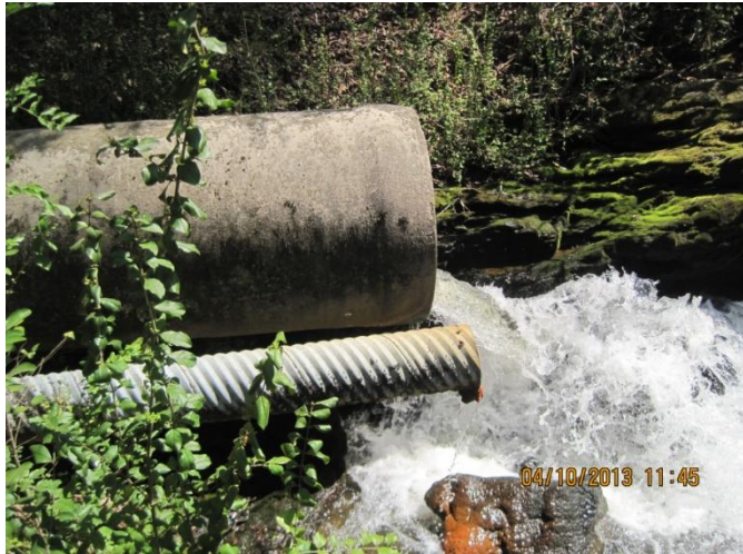
Toe drain and main outlet pipe
