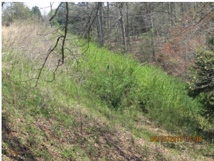
Downstream slope of dam- thick vegetation
