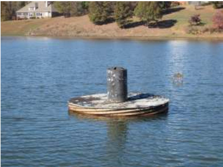
Outlet pipe with trash rack
