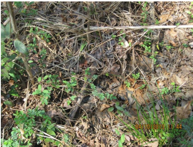
Seepage area at the toe of the dam
