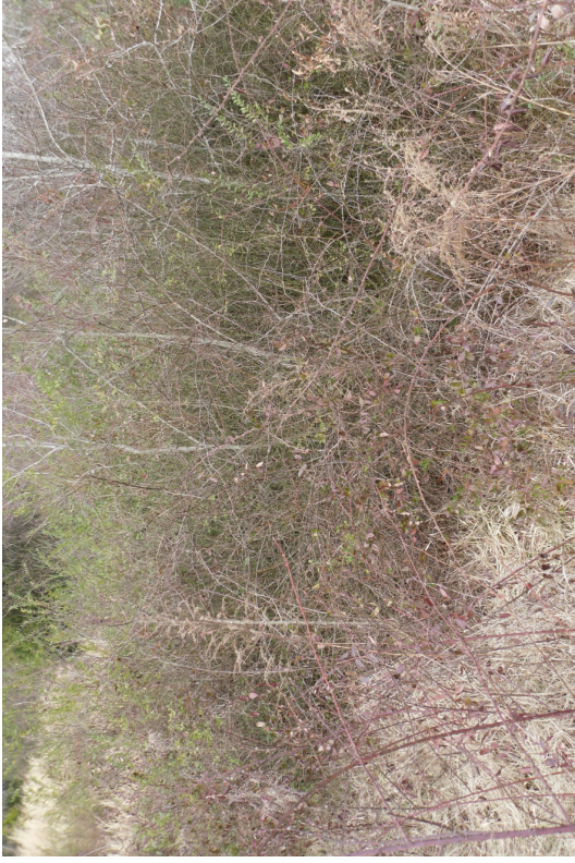
6: Thick vegetation prevented access to outlet pipe
