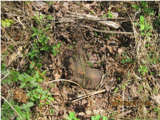
Roots on toe of dam
