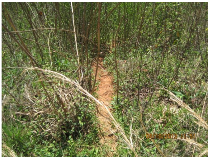
Animal trail on downstream slope of dam
