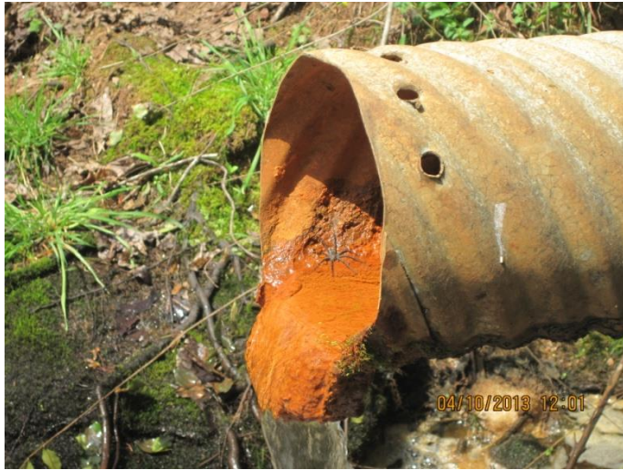
Toe drain with Iron bacteria
