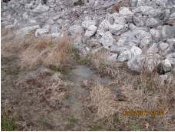
seepage at toe of channel
