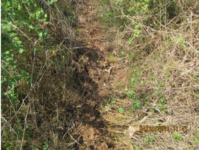
Animal trail on downstream slope of dam
