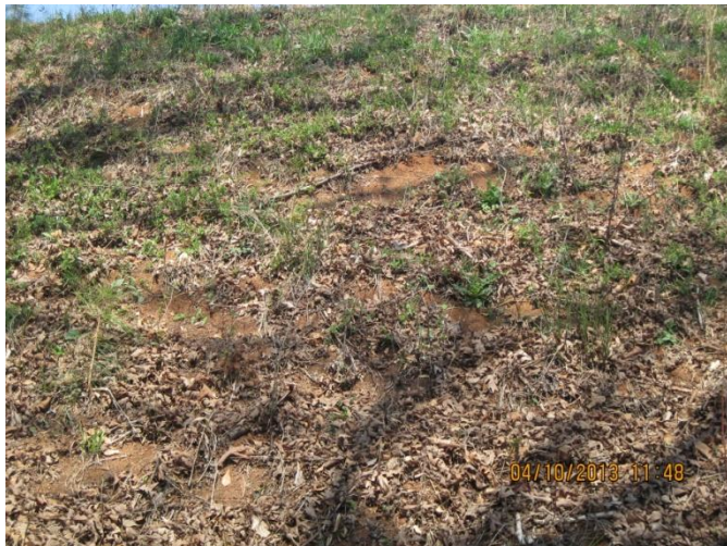
Sloughed area on downstream slope of dam
