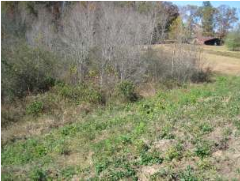
Small saplings that need to be removed around the outlet pipe.
