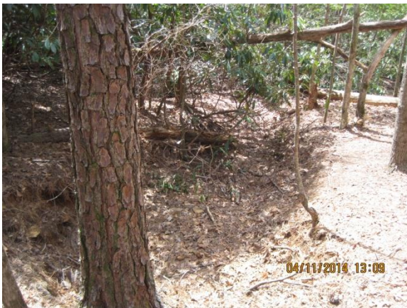
Channel being formed by emergency spillway
