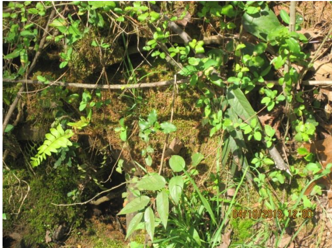
Roots at toe of dam
