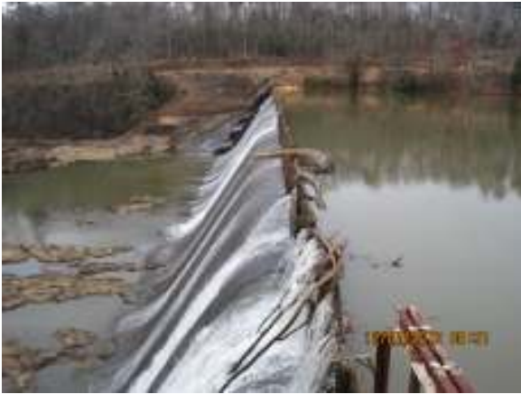
crest of dam and debris on flashboards
