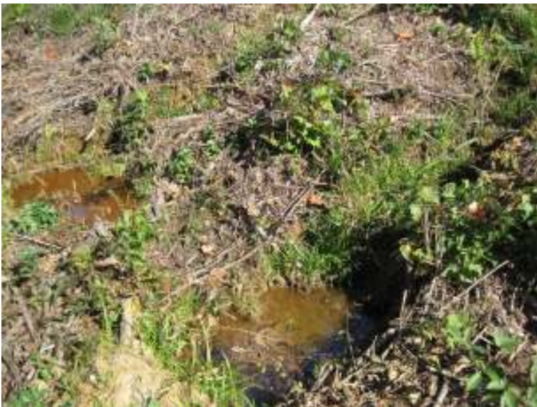
This picture shows yet another area of seepage on the down stream slope of the dam.
