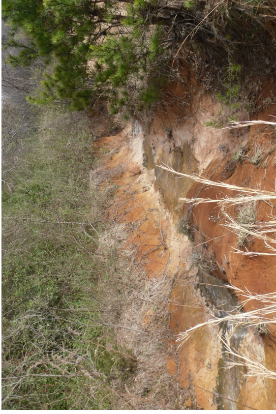
3: Significant erosion observed in the emergency spillway
