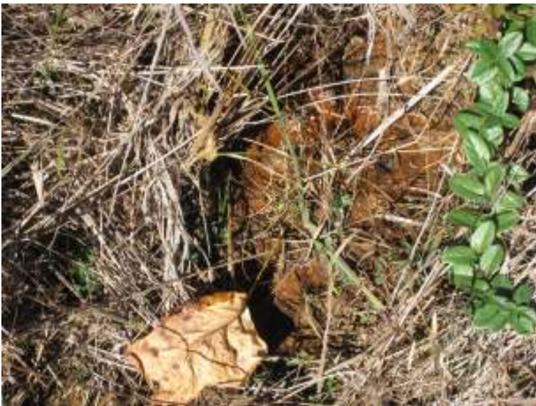
This picture is of an area of concern that shows seepage on the down stream slope of the dam.
