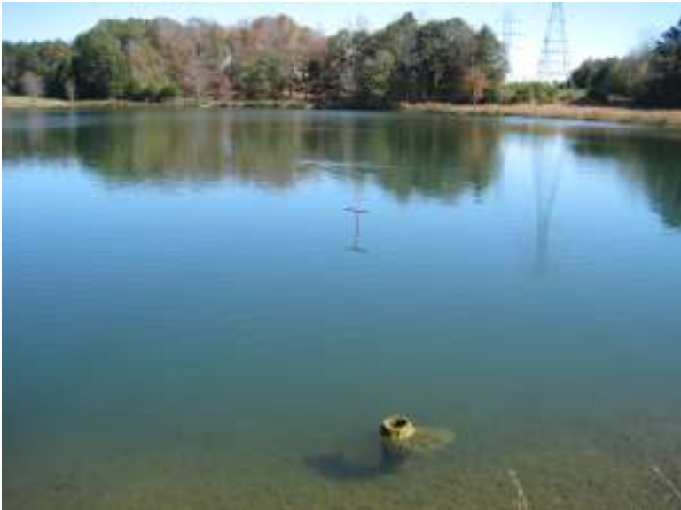
The trash rack has fallen off of the drainpipe. It can be seen to the left of the pipe in the above picture.
