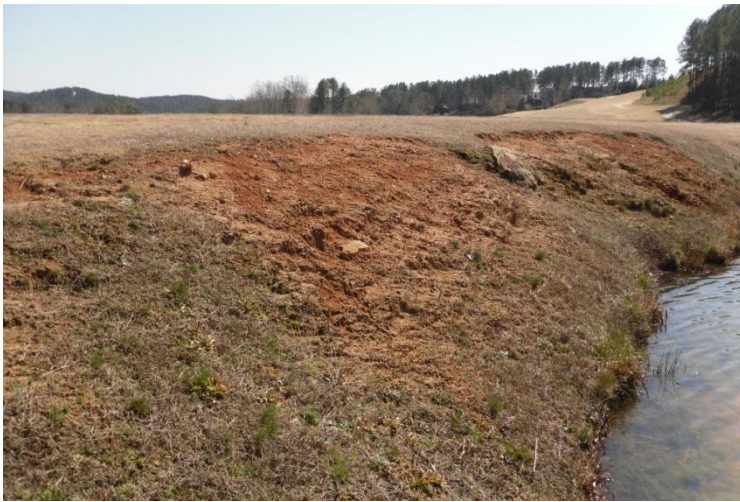
Upstream slope- needing to be stabilized
