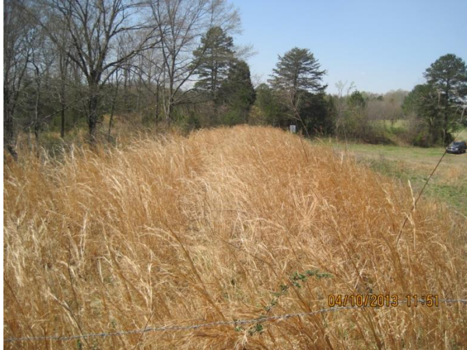
Crest of dam w/ vegetation needing to be cut
