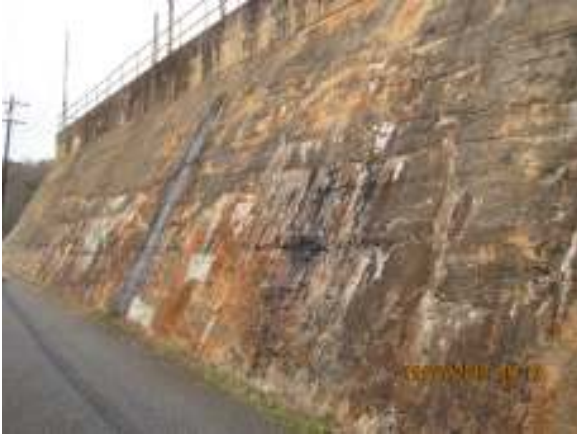
seepage at concrete structure
