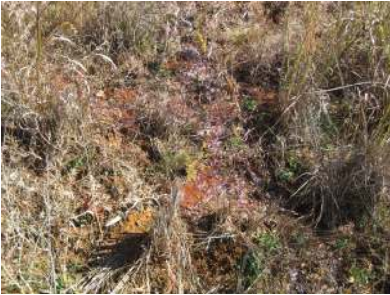
This picture is of an additional area of seepage on the down stream slope of the dam.
